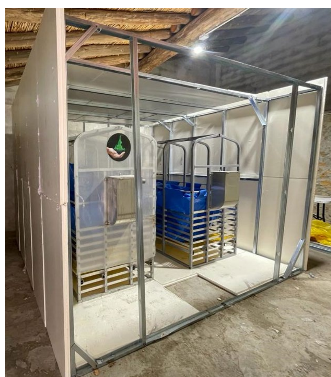
Fig. 3. Thermally insulated enclosure where the digesters are located
