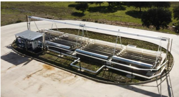
Fig. 1. View of the solar plant.
