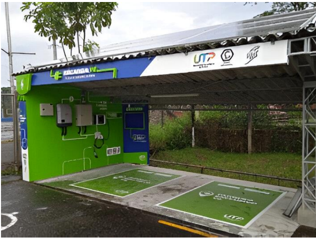
Fig. 5. Final Presentation of PV electric charging station
