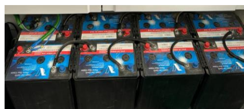
Fig.5. Batteries installed at GEDERlab.
