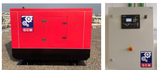
Fig.3. Diesel Generator for Biogas Simulation (Left) and Control Panel (Right).
