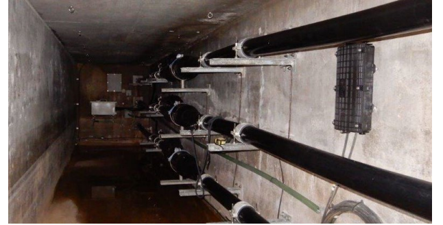
Fig. 3. Cable arrangement in junction chamber 1 (labelled CE1 and boxed in red in Fig. 2).
