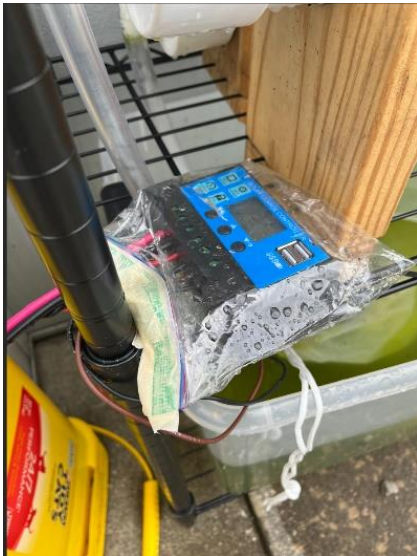
Fig. 5. Battery control module (covered to prevent rain damage)
