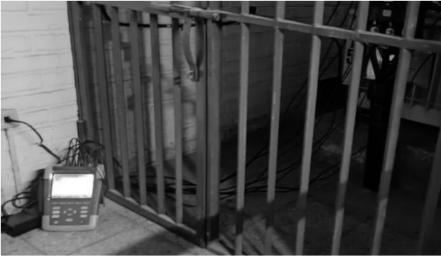
Fig. 1 Monitoring and registering power and other variables with FLUKE 345 equipment in the electrical transformer that feeds buildings, during ten days (authors)
