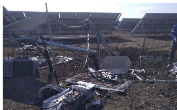
Fig. 1. Example of damaged power engineering infrastructure during the Ukrainian war.
