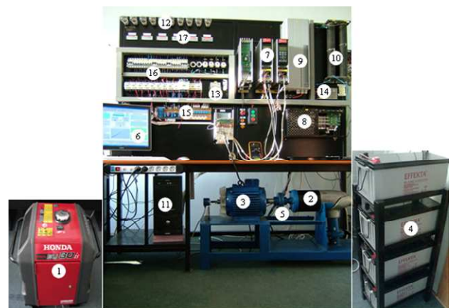
Fig. 3. The experimental rig: 1 – diesel engine; 2 – PMSG; 3 – asynchronous motor; 4 – batteries; 5 – wind shaft; 6 – software (Matlab/Simulink®, ControlDesk®); 7 – frequency converter; 8 – Whisper controller; 9 - inverter; 10 – DC load; 11 – workstation with dSPACE® board; 12 – AC load; 13 - Flexcharge controller; 14 – power supply for transducers; 15 – current and voltage transducers; 16 – circuit breakers, fuses; 17 – measurements units.
