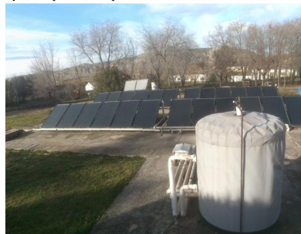
Fig. 1 Solar collectors and storage tank's overall view.
