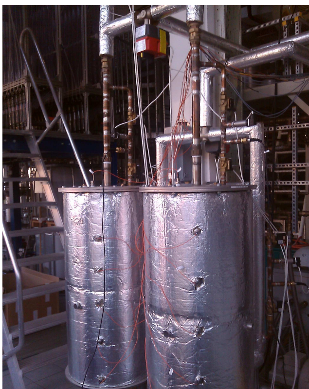
Fig. 10. Zeolite exhaust gas condenser.
