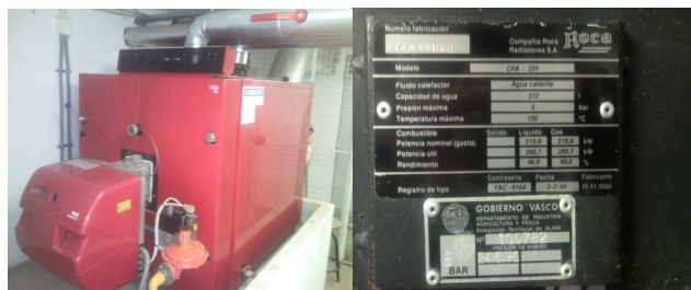
Fig.7. Existing boiler and control panel.
