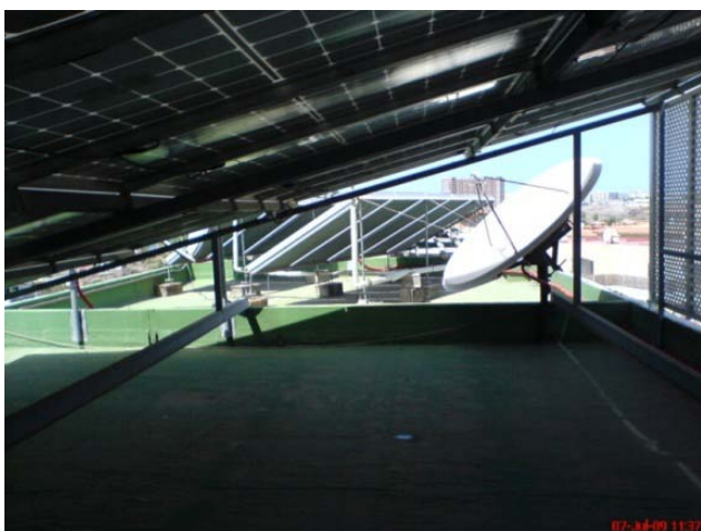
Fig. 1. Photovoltaic power plant
