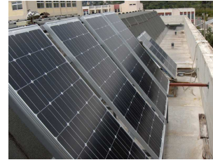
Fig. 2. P/V bank on the roof of E.C.L.
