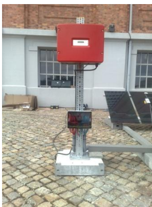
Fig 7. View of the Solar Inverter
