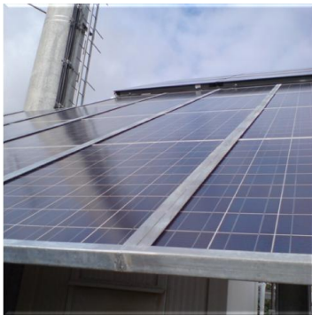
Fig 6. View of the solar panels
