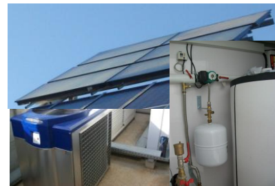
Fig 14. Some of the solar cooling systems equipments [4]
