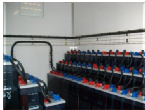
Fig 10. Bank of batteries
