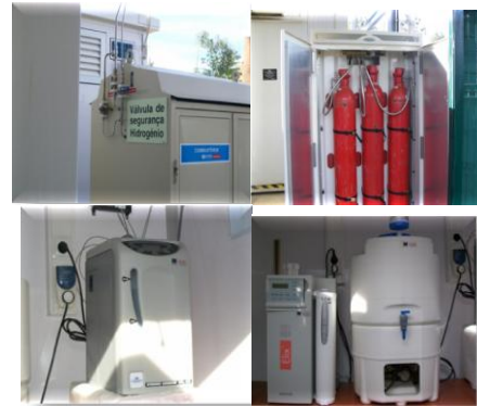
Fig 13. View of the hydrogen production equipments
