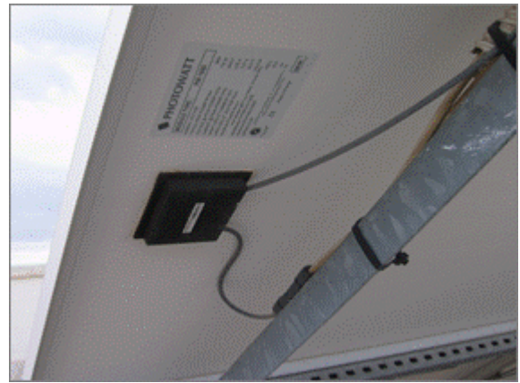
Figure 3. The connection box.
