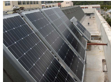
Fig. 2. P/V bank on the roof of L.E.M.E.C
