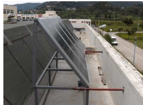
Fig. 8. Metallic base of PV-panels with a mechanism to change the slope, on the roof of L.E.M.E.C.
