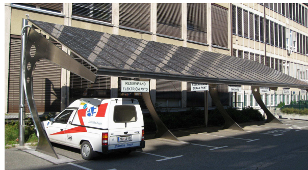
Fig. 1. Photovoltaic (PV) system installed at University of Maribor.
