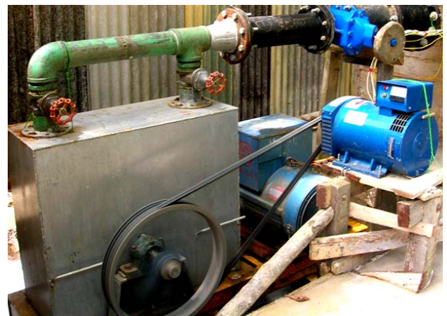
Fig. 5: Final setup of the 30 kW turbine generator.
