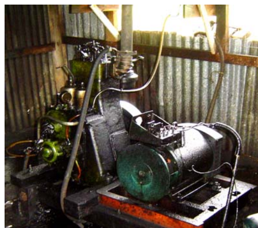
Fig.1: Diesel generator set in a remote village.
