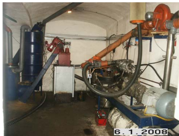
Fig. 2. The plant at January 2008.
