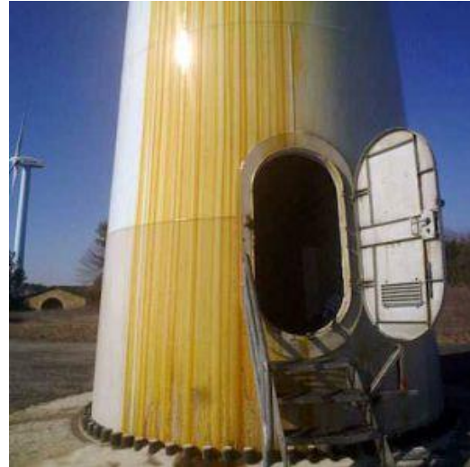
Fig. 11. Oil leak along a wind turbine tower in the Sierra de El Perdón [15]
