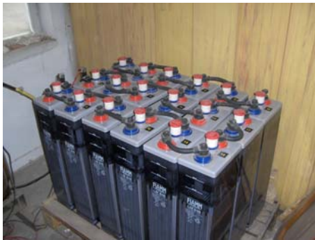
Figure 9-Batteries used as load
