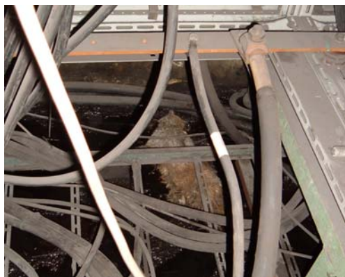
Photo 1. A cat corpse inside an electrical cabinet.
