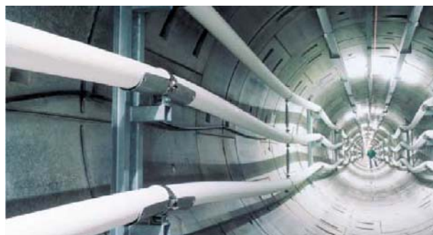
Figure 1. Underground power line
