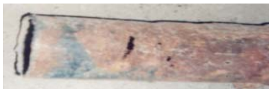
Fig. 2. Corrosion of a gas pipeline due to the a.c. and d.c. dispersion currents
