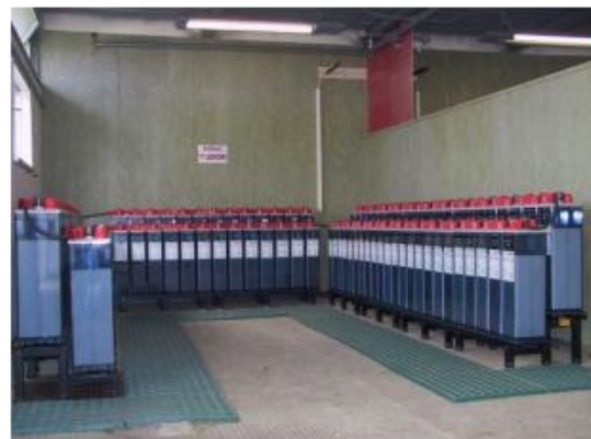
b) Battery room
