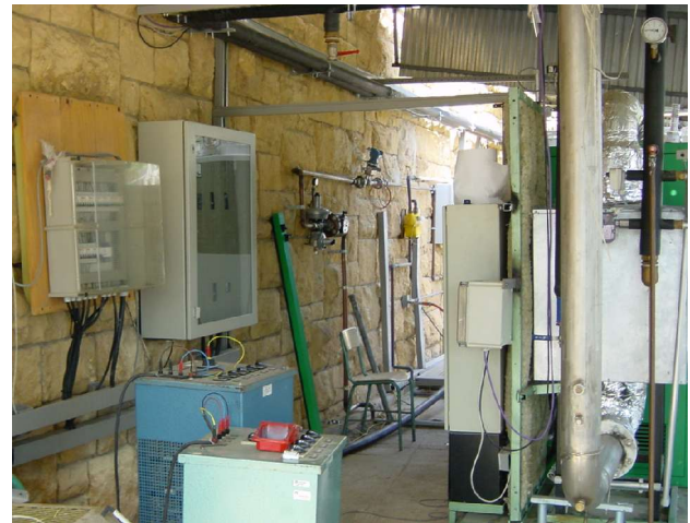
Figure 2. View of the micro gas turbine test facility in CREVER-URV (Tarragona).
