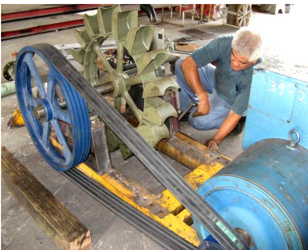
Fig. 4: 30 kW homemade turbine generator
