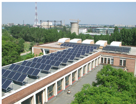
Figure 1. General view of double array 30 kWp PV grid-connected demonstration system.
