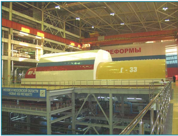
Fig. 1. Asynchronous turbogenerator of 160 MW on the Moscow Power Station
