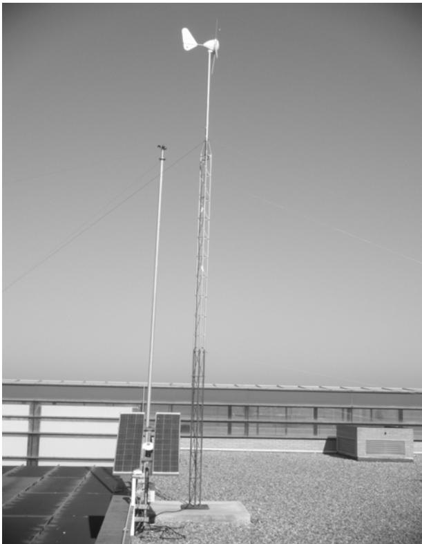
Figure 3. Wind – solar generator
